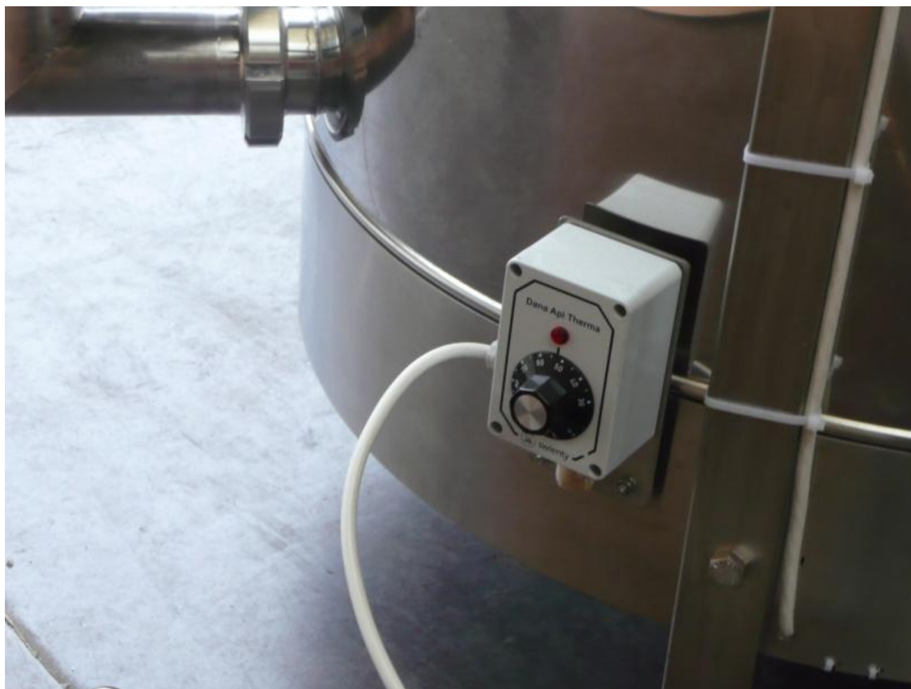
Image 5: Thermostat floor heating
